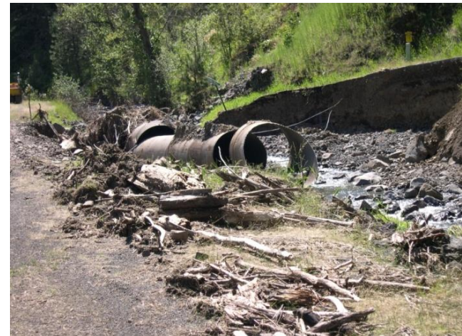
Figure 22. Culvert and stream damage after a flash flood, 2010. Photo: Casey McCormack.
