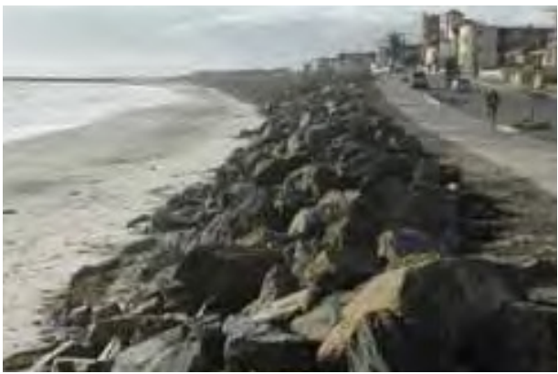
Australian Government: Climate Change Risks to Australia's Coast A First Pass Assessment, 2009 Figure 6: Rock seawall along Adelaide's West Beach
