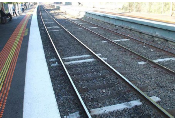
Source: Courtesy of Ifte Ahmed. Figure 5: Timber sleepers are being replaced by concrete sleepers to resist track buckling due to high temperatures
