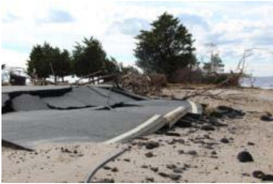
Figure 4. Coastal road destroyed by overwash. (credit: Amanda Babson and Courtney Schupp, National Park Service)
